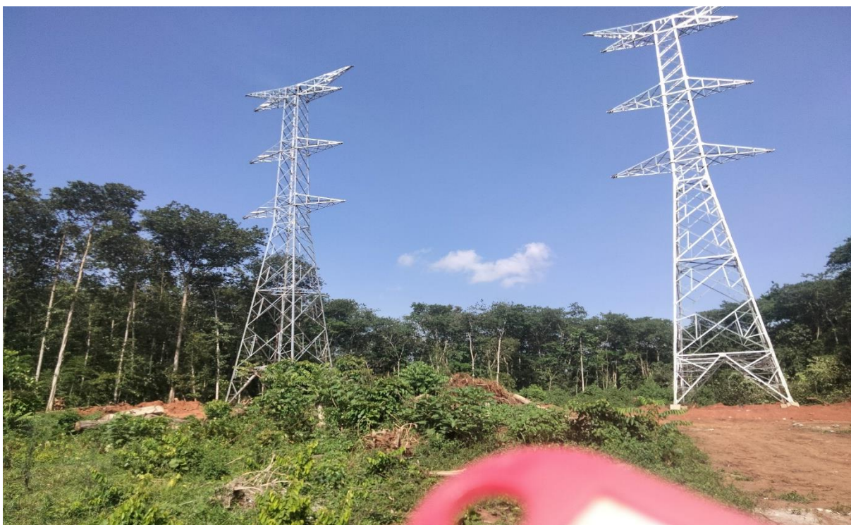
Picture 2: Completed Angle Tower 3 pending Stringing 132kV and 220kV transmission lines in Nandagi Reserve Forest.
