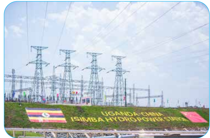
132KV Isimba Switchyard
