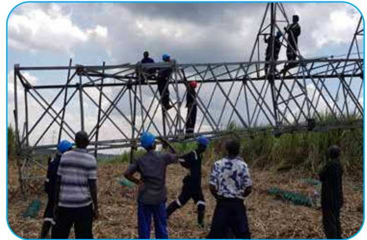
Inspection of a vandalized transmission tower
