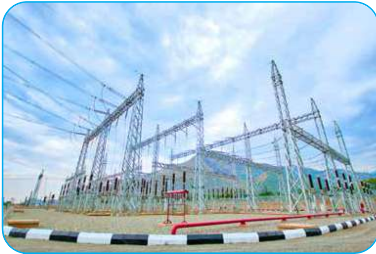
220 / 132kV Nkenda Substation
