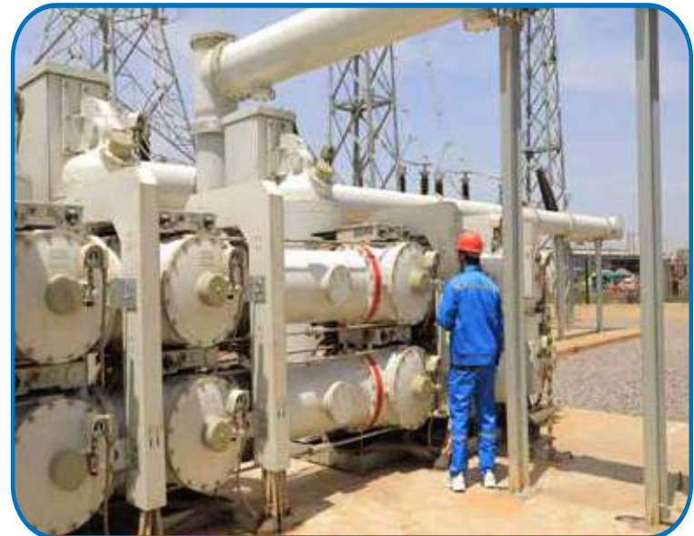
Namanve South 4 Sub Station
