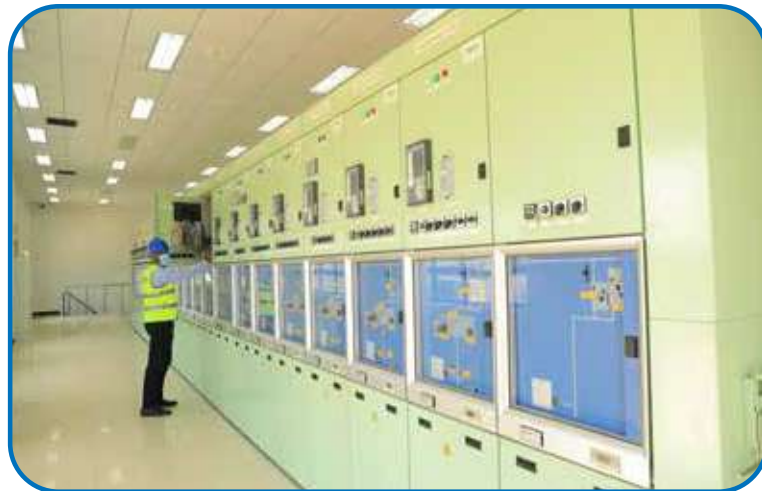
Namanve South 2 substation
