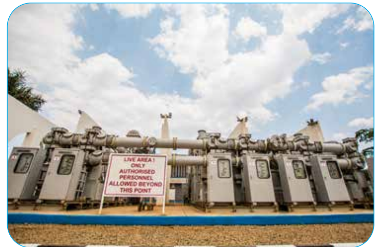
132/33 KV Queensway Gas Insulated Substation (GIS)
