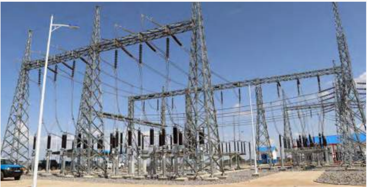
▲ The new Moroto Substation
