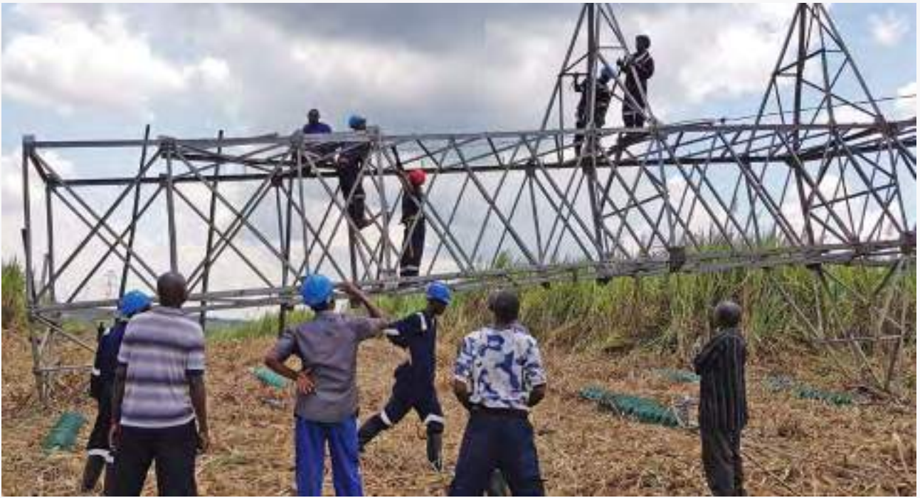
▲ Collapsed Tower after vandalism
