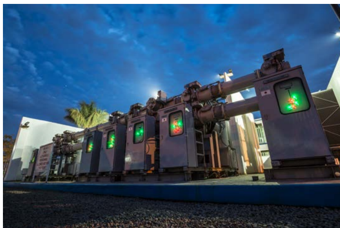
132/33kV Gas Insulated Substation
