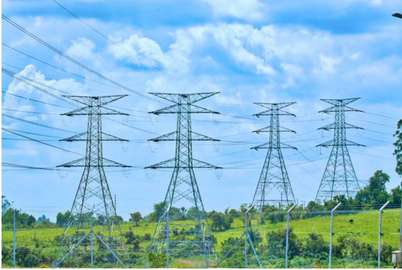
Fort Portal 132kV transmission power lines
